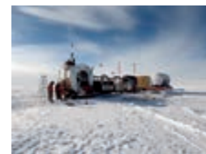
Drilling holes for ARA construction using a particular drill machine. (from ARA website)
