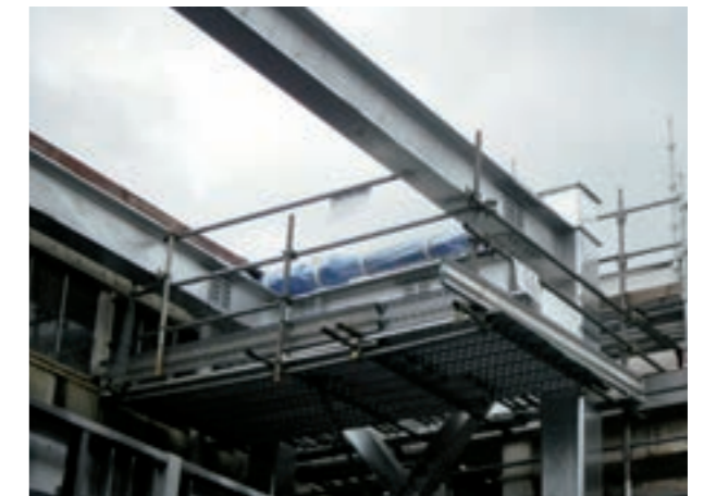
Seismic control devices were placed on the external part of a building, thus people were able to continue their operation as usual.
